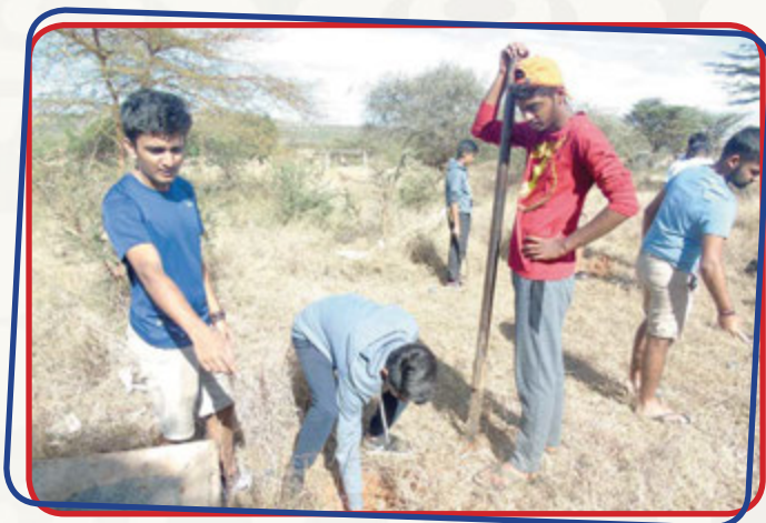
Team Work: Manthan and Geo help erect a rubbish pit perimeter fence.
